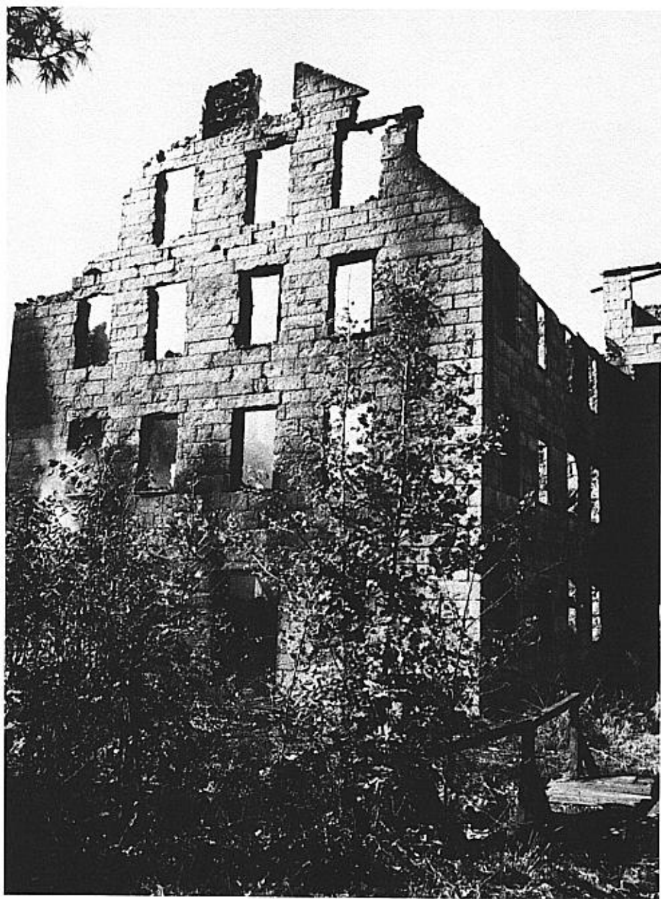
CROWN AND EAGLE MILLS, North Uxbridge, Massachusetts, October 9, 1975, after a disastrous fire gutted the entire complex. (Photograph courtesy of OSV.)
